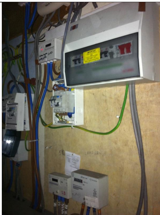
14 Cover missing on fuse board in open electrical cupboard
