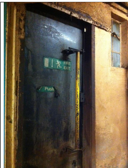
07 Rear fire exit – jammed shut
