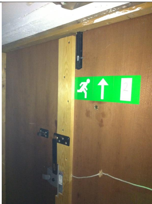
10 First floor fire exit – bolted shut
