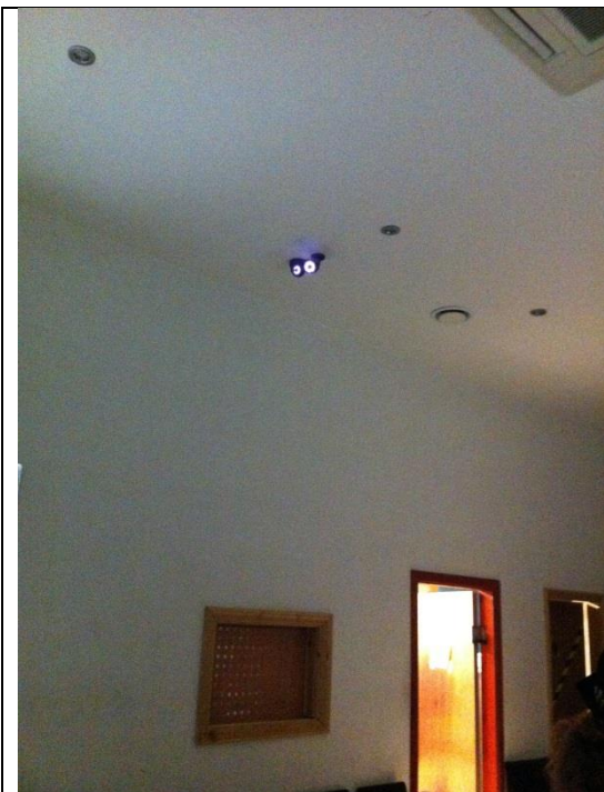
25 CCTV in the middle of shisha smoking room
